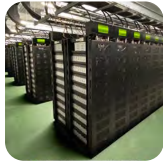
BESS Battery Energy Storage System
